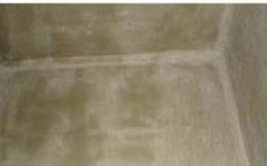
Horizontal and vertical covers using Fibre-Patch OV, Cem-Kote Flex ST and Reinforcing Fabric HD, Brantford, Ontario, Canada
