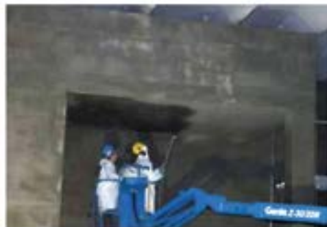
Cem-Kote Flex ST applied to walls and slab, Herridge WTP, Mississauga, Ontario, Canada
