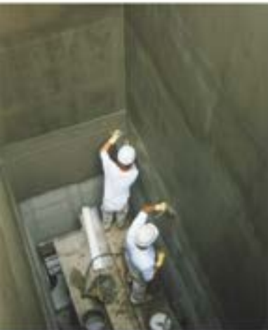
Installation of Cem-Kote Flex ST with Reinforced Fabric HD throughout (entire surface), Kingsford, Ontario, Canada
