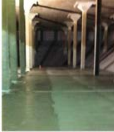
Cem-Kote Flex ST in restoration and waterproofing of Whaley WTP, Vancouver, British Columbia, Canada
