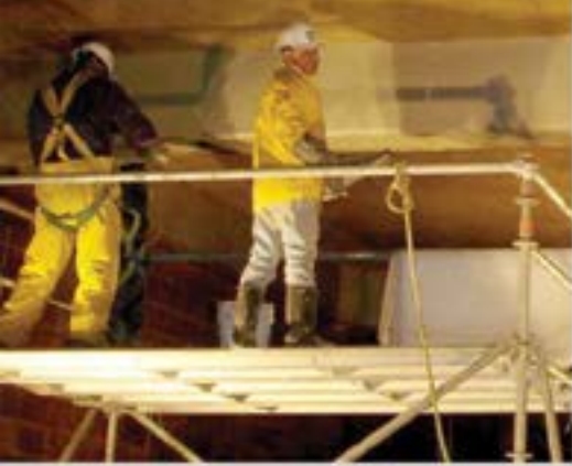
Cem-Kote Flex ST and Reinforcing Fabric HD applied over a high number of cracks in the beam, Guelph, Ontario, Canada
