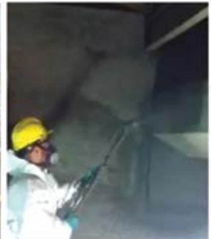
Spraying of Gem-Plast TC to repair and level deteriorated concrete surface, Niagara, Ontario, Canada
