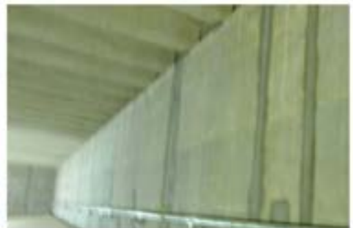
Cem-Kote Flex ST with Reinforcing Fabric HD to provide long term crack bridging, Mississauga, Ontario, Canada
