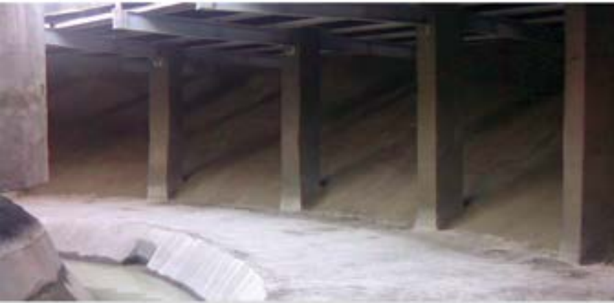
Cem-Kote Flex ST used to restore and waterproof WTP in Calarasi, Romania
