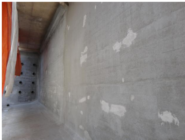
Figure 2. Cem-Kote Flex ST applied to the walls of one of the several tanks.
