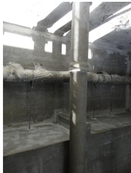
Figure 3. Steel pipes were rust-proofed using Fibre-Prime and then coated with Cem-Kote Flex ST.
