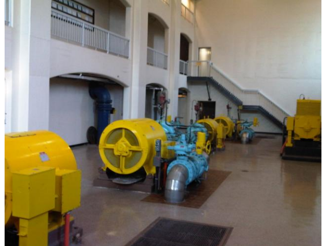
Figure #1. The mechanical part of the facility
