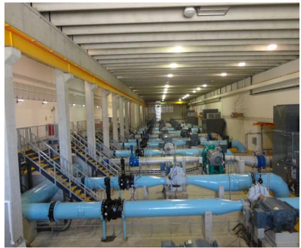
Figure #1. The mechanical part of the facility
