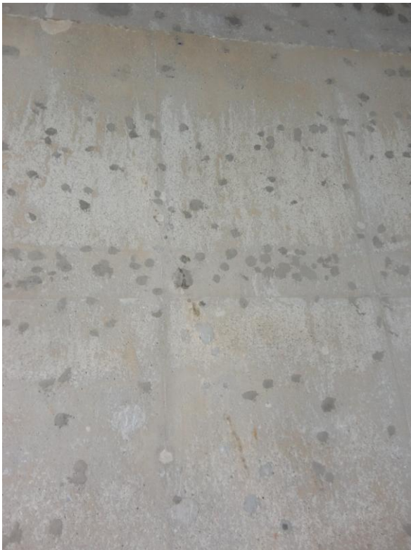
Figure #6. Parging the “bug holes” (dark spots) in the tank 1B using Gem-Plast TC
