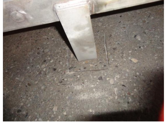
Figure #5: Near perimeter cuts to provide an interlock for Cem-Kote Flex ST terminations
