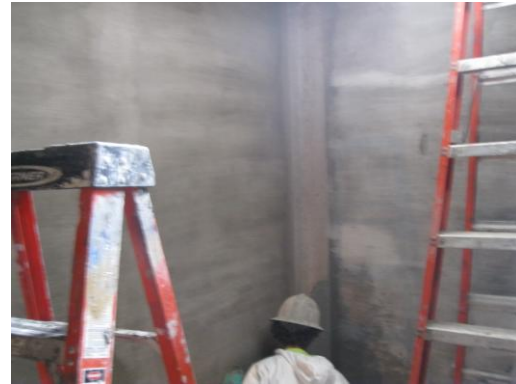
Figure #1: Interior of the tank at Bay Bulls – Cem-Kote Flex ST application
