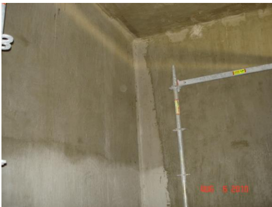
Figure 6. Refurbished chlorine treatment tanks to ozone treatment. Initial installation in 1998, modification in 2010
