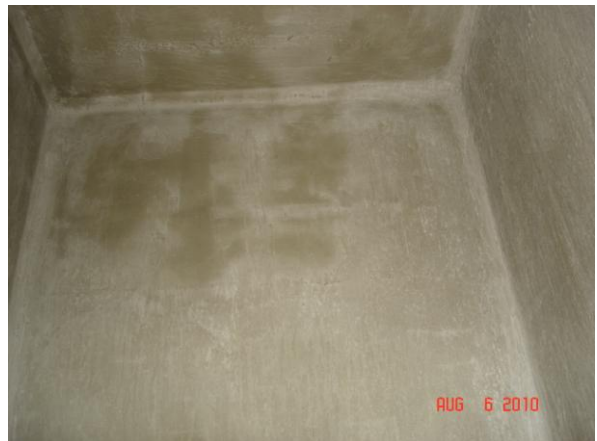
Figure 7. Refurbished chlorine treatment tanks to ozone treatment. Initial installation in 1998, modification in
