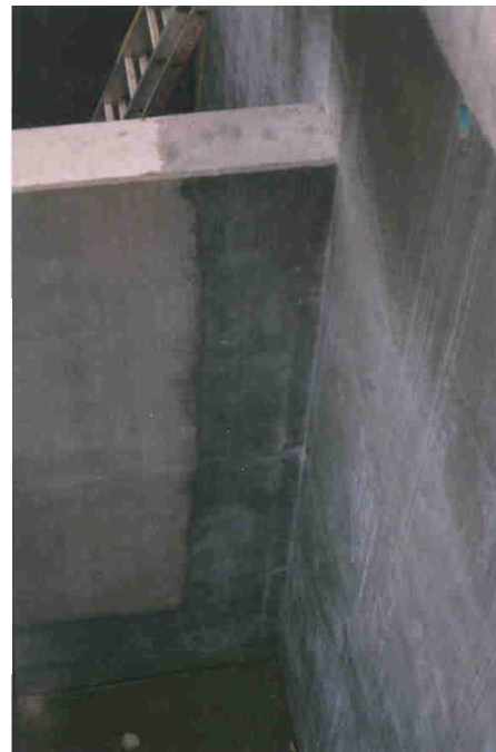
Figure #3. The same as the area shown in Figure #2. The black area to the left is concrete covered with carbonated sludge, in the middle is clean concrete surface and to the right Cem-Flex ST marked by stream of high pressure water.
