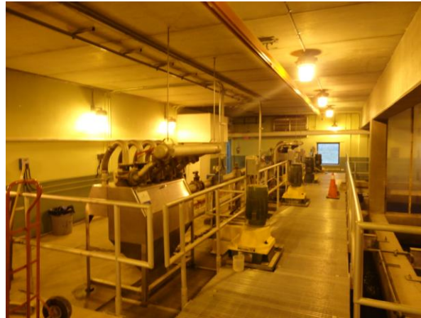
Figure #1: top of tanks showing the sand cleaning and recycling equipment
