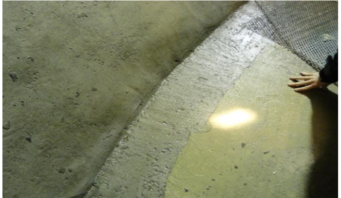
Figure #5: the bottom of the Tank #3. Cleaned Cem-Kote Flex ST to the right, the removal required water pressure in excess of 12,000 psi.
