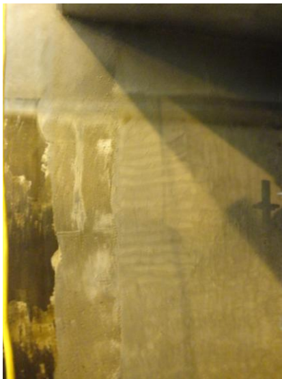
Figure #2: Cem-Kote Flex ST waterproofing applied to exterior wall of the tank #2 and partly on partition wall separating tanks #1 and #2
