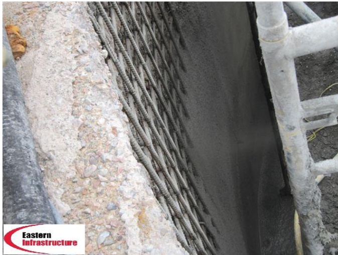
Figure 4. Application of Spray-Con WS ST, wet shotcrete, to repair concrete sections. Spray-Con WS ST was supplied as concentrate, and mixed with cement water and aggregates, according to mix design supplied by Gemite, in the near batch plant. The first batch was 2 cubic meters, the following batches were supplied in mixing truck by 3 cubic meter sizes.
