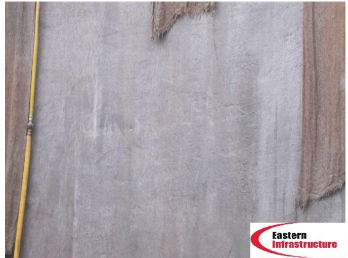
Figure 5: Spray-Con WS ST repair. The entire surface of the tank was coated with Cem-Kote Flex CR within 2-3 days after application of Spray-Con WS ST
