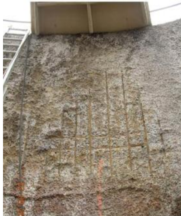
Figure 1: concrete deterioration taking place between 2003 and 2010, after the placement of roof in 2003.
